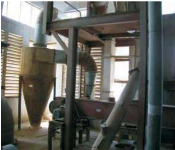
Fig 5.19-Proper dust extraction system with cyclone and ID fan in Large mills
