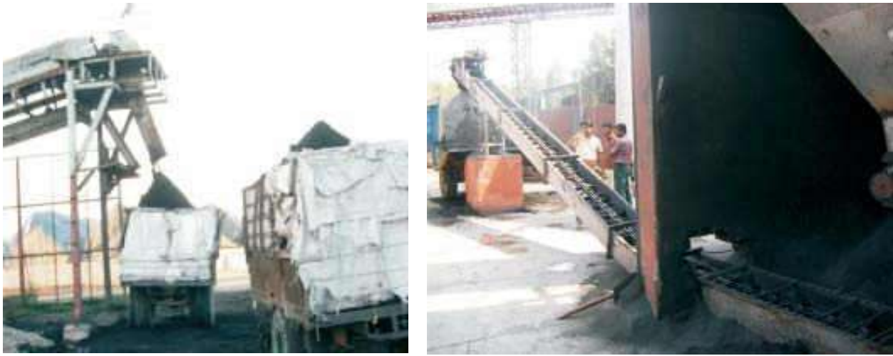
Fig 4.13-Mechanical handling of boiler ash
