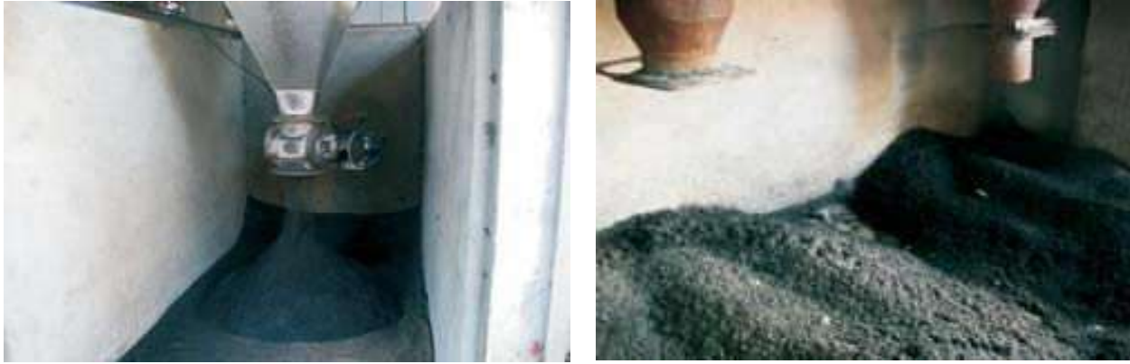
Fig 4.16-A Closed storage of husk fired boiler ash
