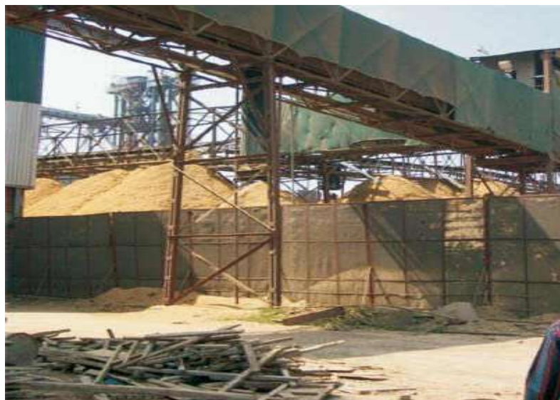
Fig 4.11-Husk Handling from storage yard to boiler using conveyor belts in large mills
