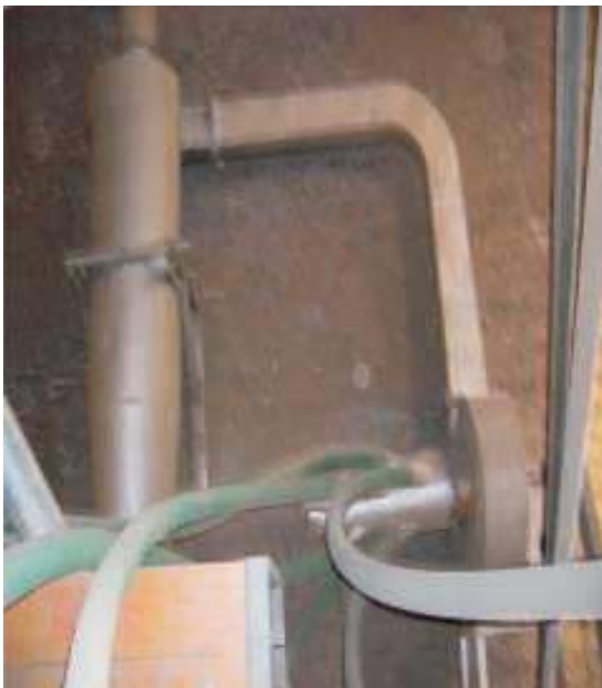
Existing Dust Extraction cum Control System
