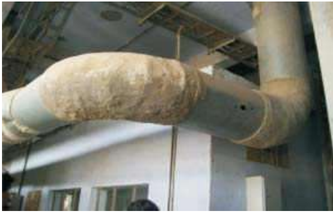
Fig.6.7. Common Duct from Paddy Separators (2 nd floor) (Port Hole 10)
