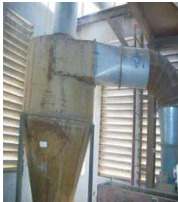
Fig.6.10. Cyclone Inlet (Port Hole 7) on 4 th floor
